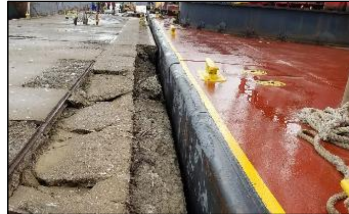
20' failed section of the lock chamber wall (13 APR 2018)
