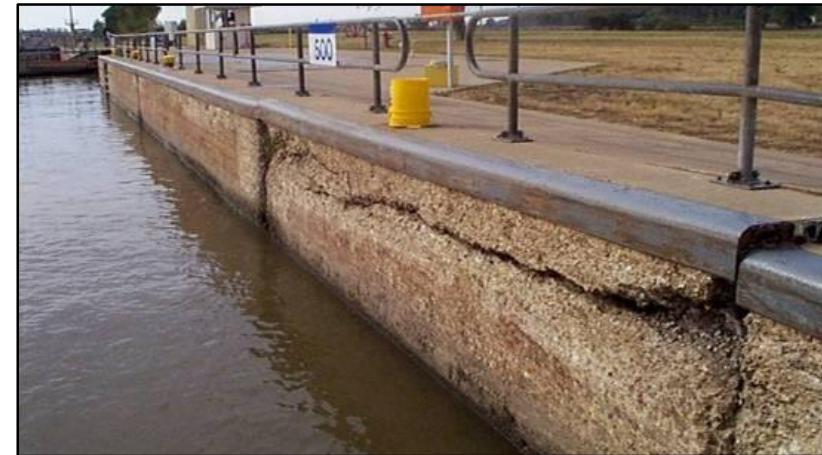
Unsafe conditions for both lock workers and the Navigation Industry
